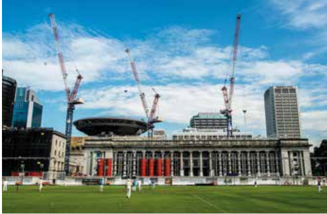
Above: Linden Comansa luffing-jib cranes being used on the National Art Gallery project in Singapore.
