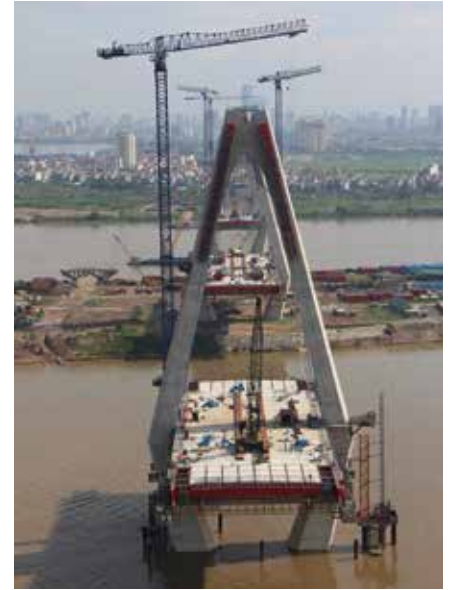
Linden Comansa flat-top cranes at work on the Nhat Tan Bridge project in Hanoi, Vietnam.
