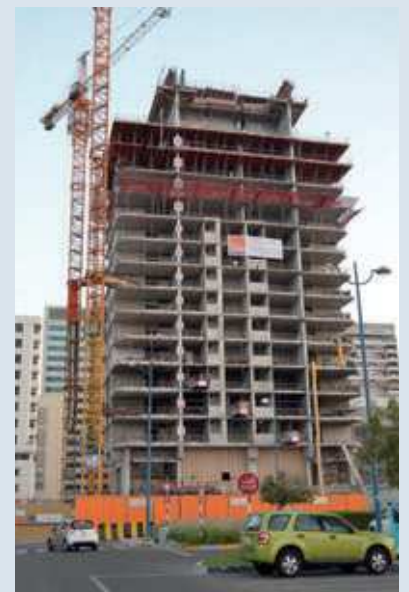
RMD Kwikform played a part in residential and commercial Al Jazeera Tower, Abu Dhabi
